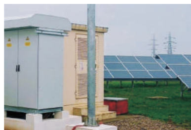
Energy Storage Cabinet
